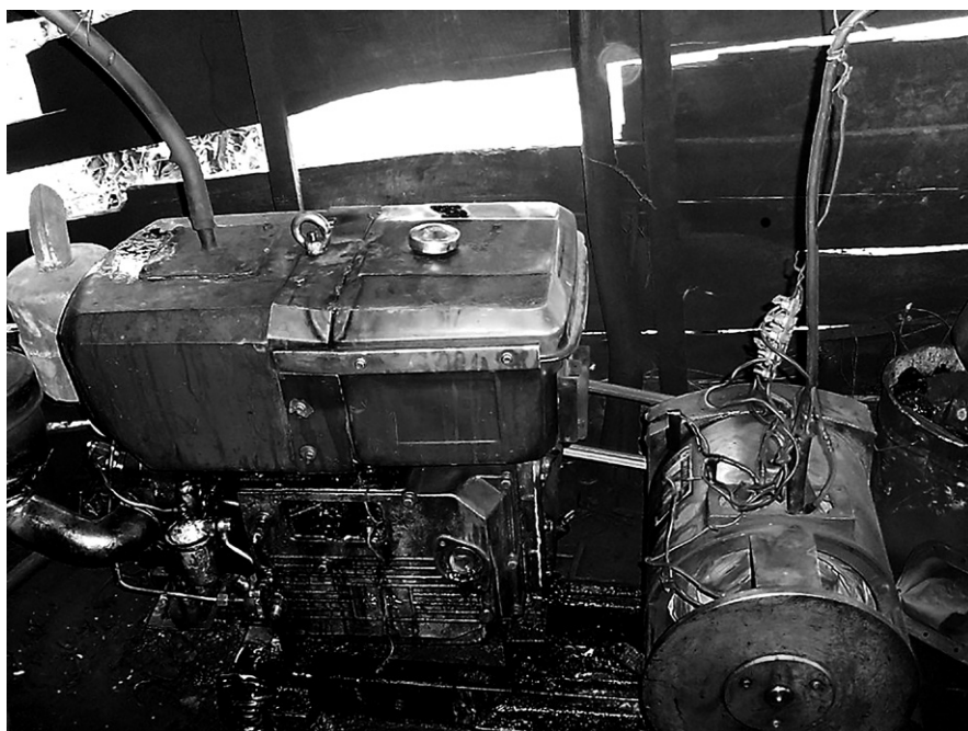
Figure 6.4 Commercial generator, photographed 2 August 2014, Keshero, Goma
